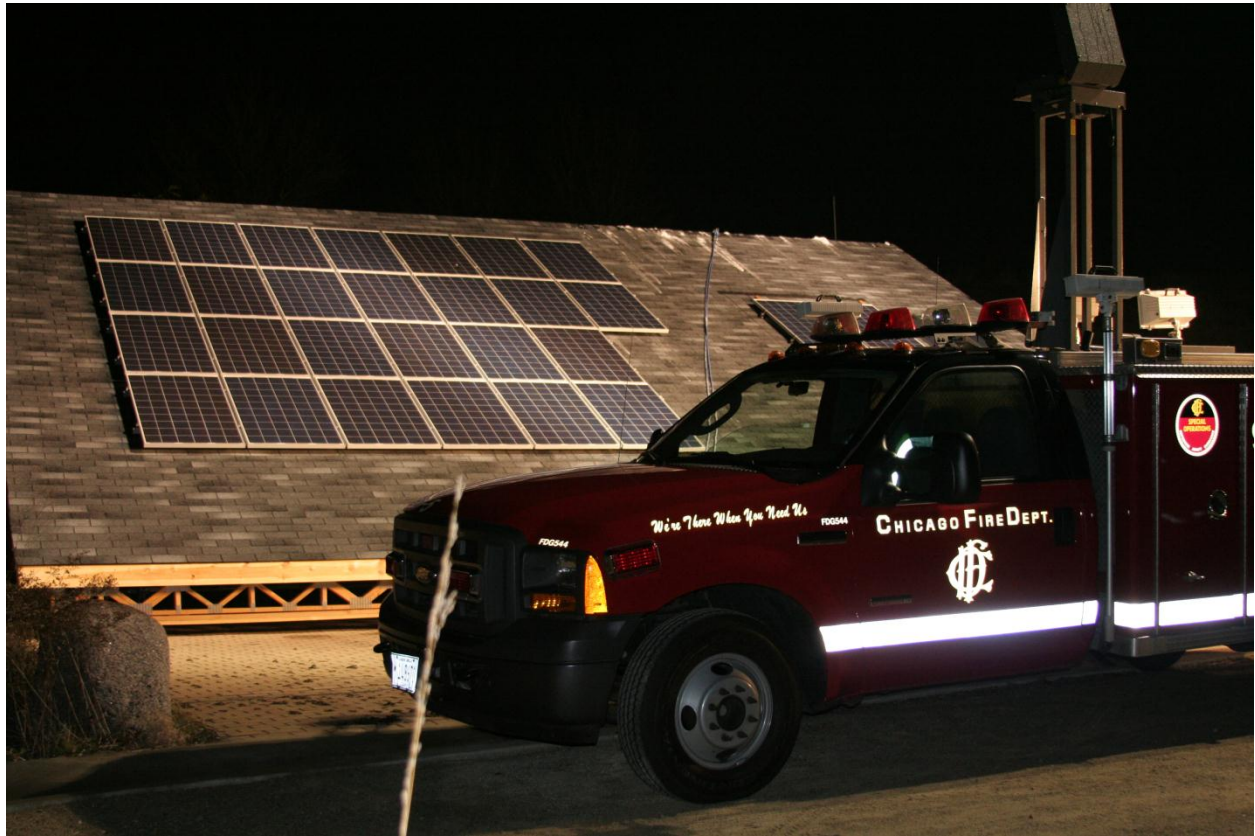
Figure 70 - Array being illuminated by Light Truck No. 1
