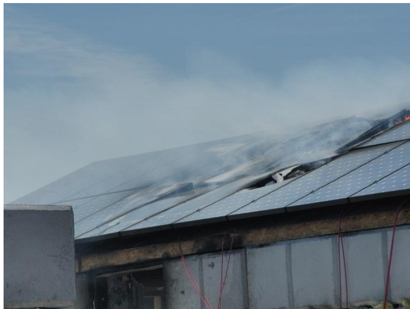
Figure 191 Broken glass and debris
