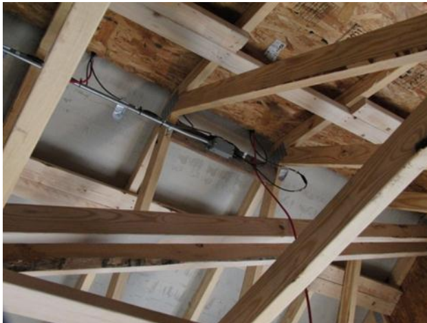
Figure 92 Laminate lead wires and home run
