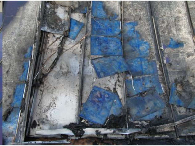
Figure 137 Exposed bare lead wires
