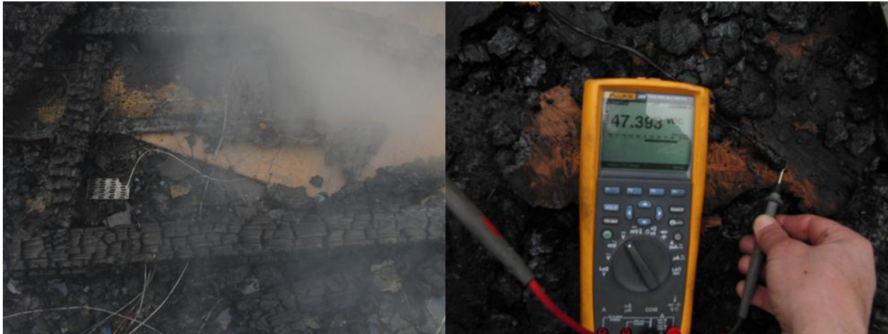
Figure 156 Exposed lead conductors in rubble Figure 157 Voltage between exposed wires
