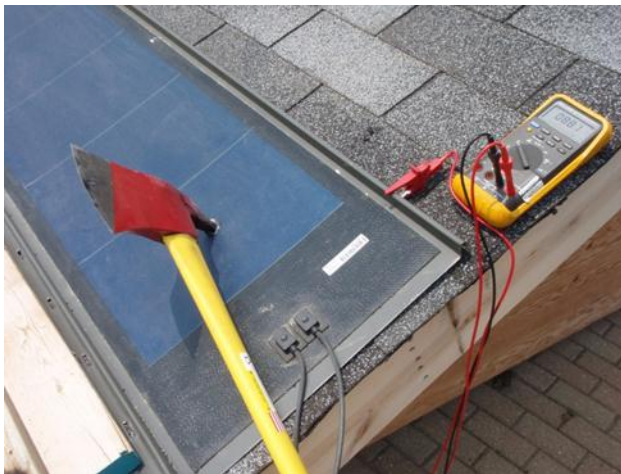
Figure 65 Axe penetrates laminate
