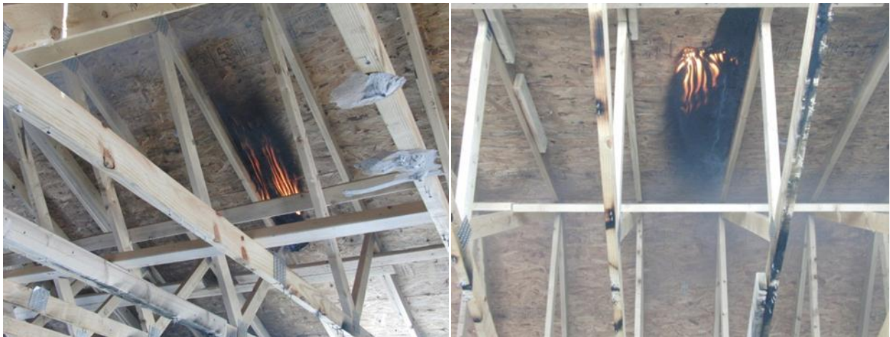
Figure 194 Flaming of underside of roof deck Figure 195 Close up of flaming
