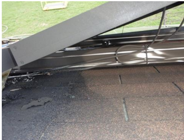
Figure 184 Looking under module for dangers
