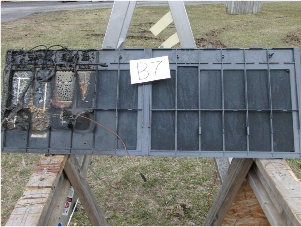
Figure 159 Shingle B7 with exposed lead conductor
