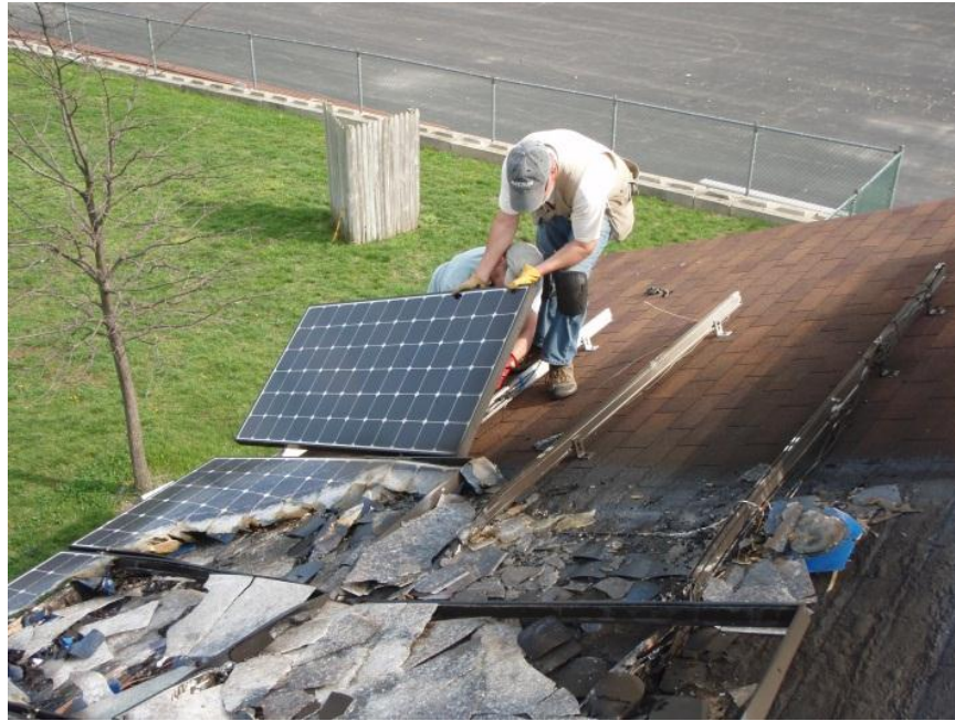
Figure 186 Work continues closer to damaged modules
