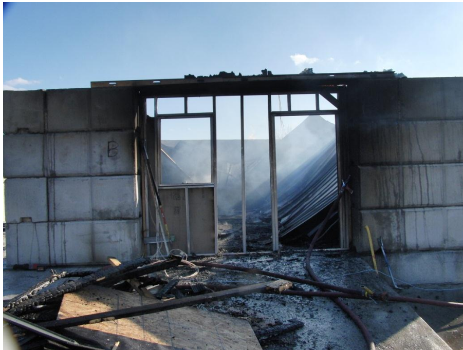
Figure 127 Collapsed roof and laminates
