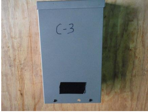
Figure 21 Combiner Box C3
