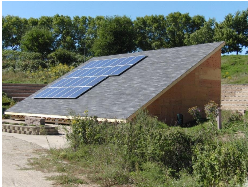
Figure 40 Main test array with 26 PV modules
