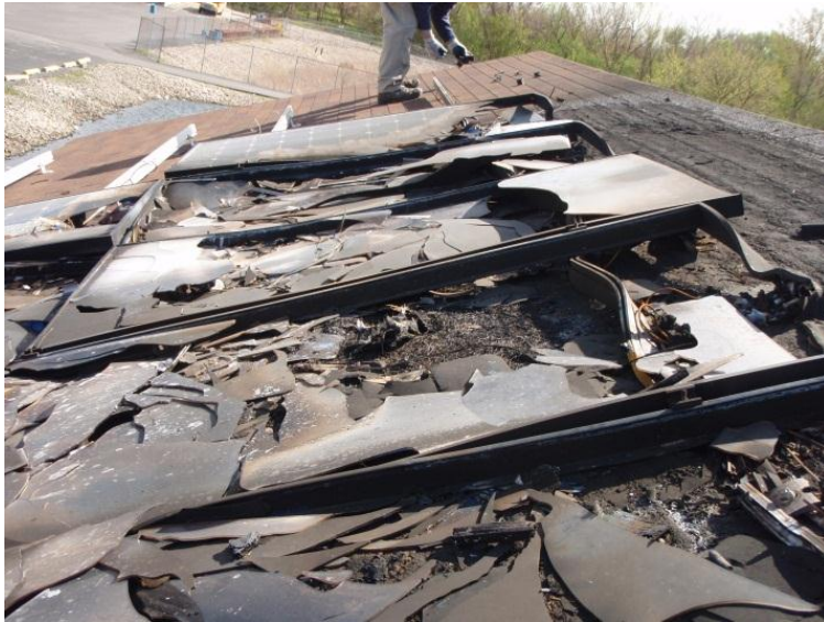
Figure 196 Destroyed modules on roof
