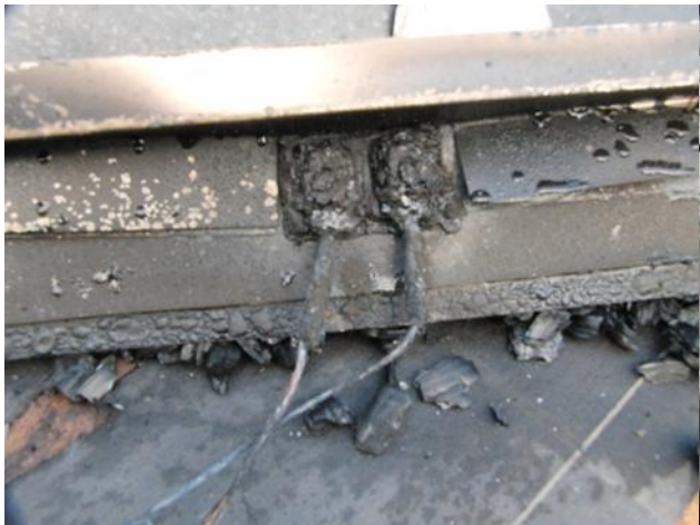
Figure 138 Exposed bare wires at junction box
