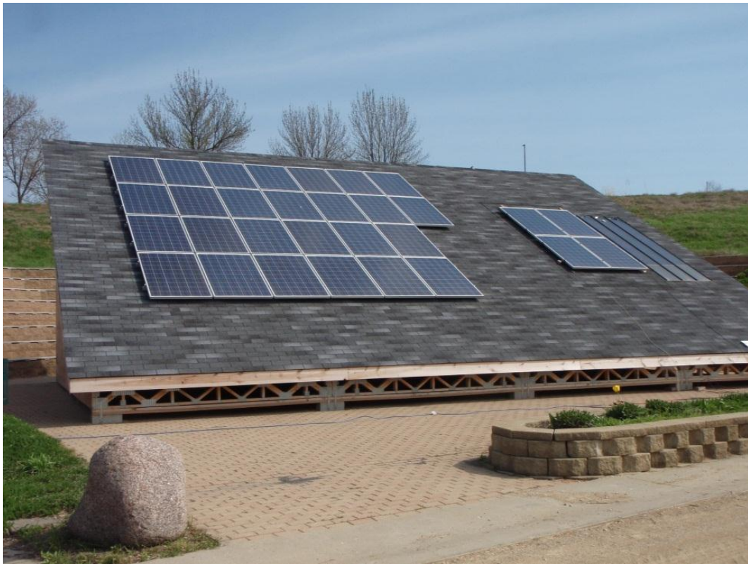
Figure 41 Complete structure with PV framed modules and laminates
