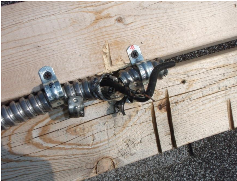
Figure 60 Exposed conductor from action of chain cutting
