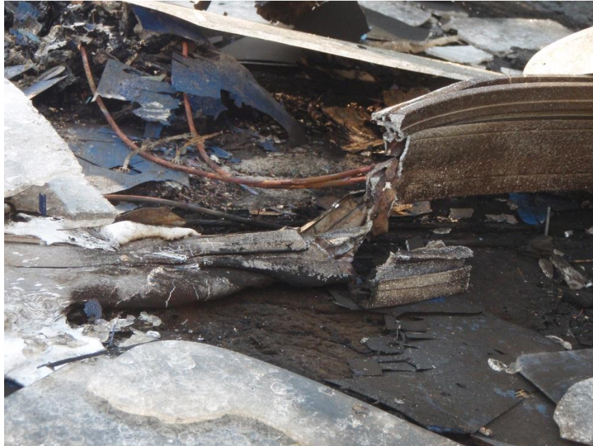
Figure 183 Bare energized conductors contacting broken rails and metal frames
