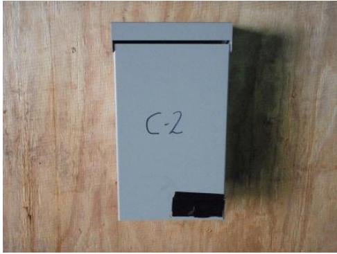
Figure 19 Combiner Box C2
