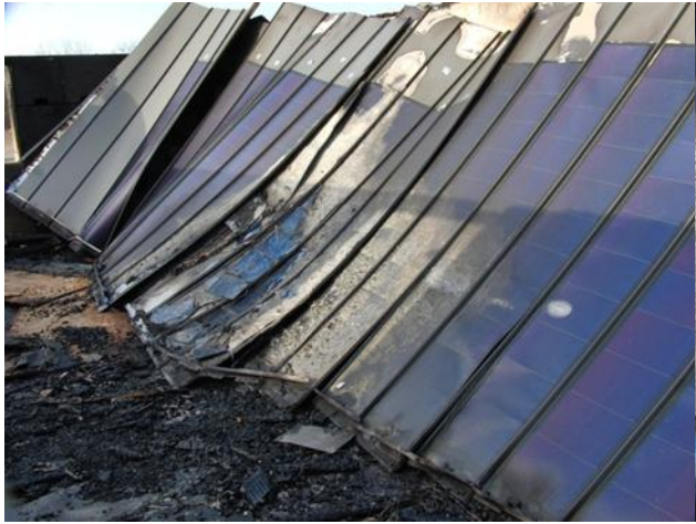
Figure 136 Collapsed and damaged laminates
