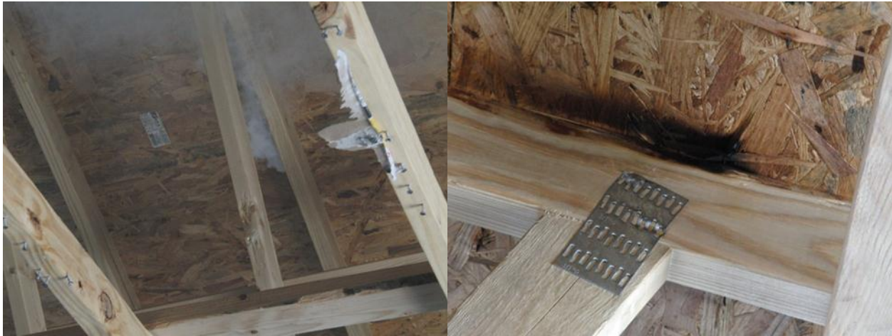
Figure 192 Smoke developing on inside of roof Figure 193 Charring on inside of roof
