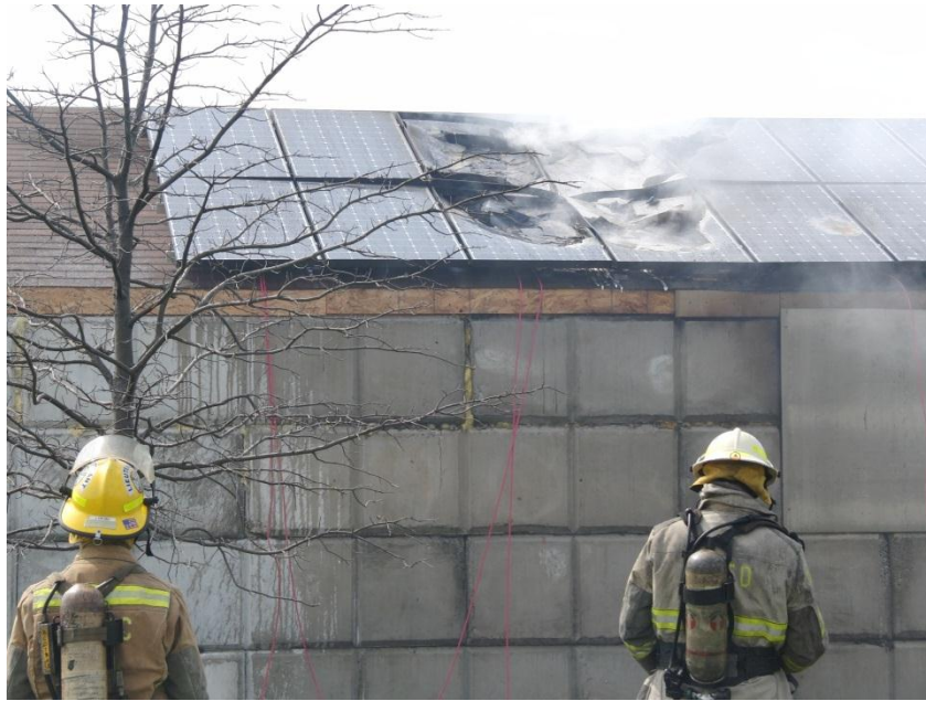
Figure 177 Firefighters assessing damage after fire
