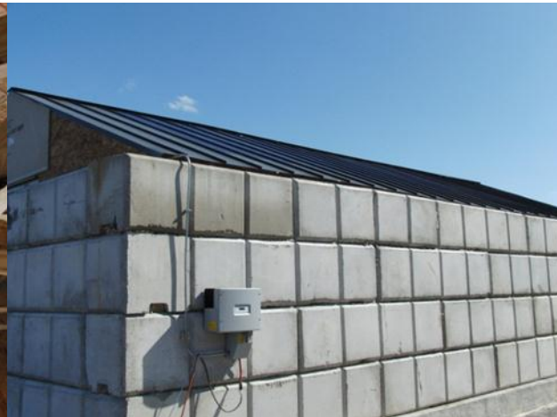
Figure 93 Inverter/disconnect near ground
