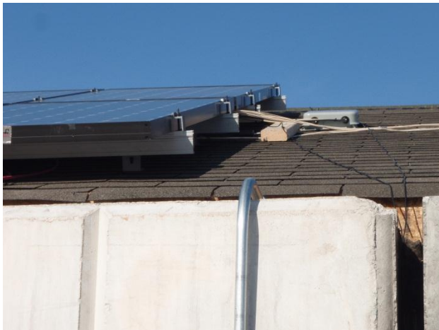
Figure 89 Modules mounted off roof / EMT to inverter
