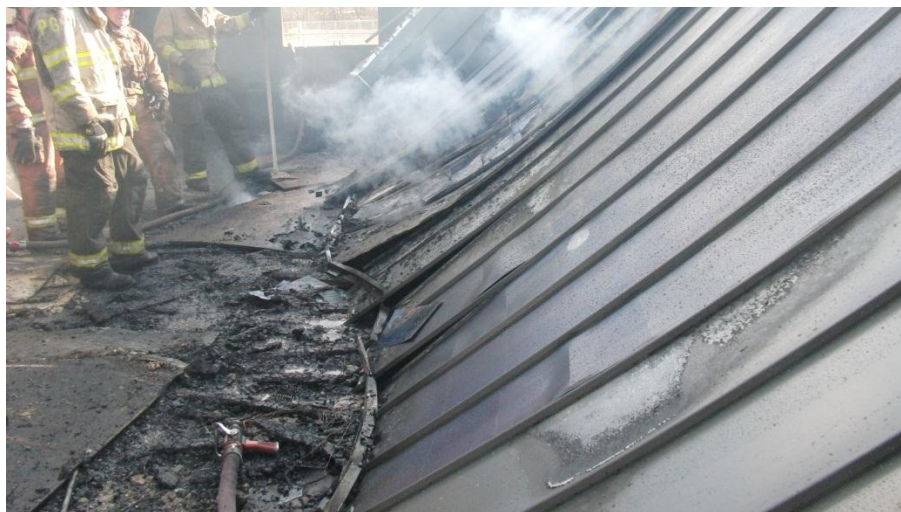
Figure 128 Firefighters approaching Collapsed Laminates after Fire
