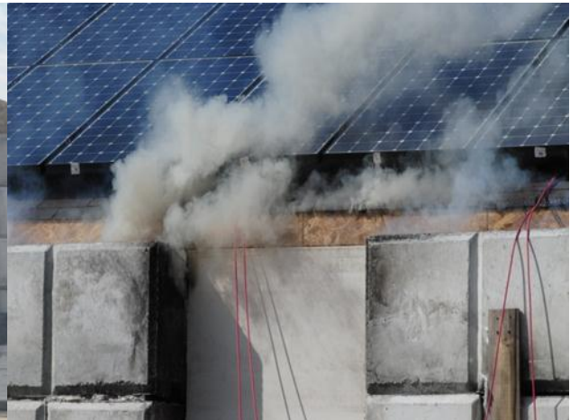
Figure 100 Some smoke coming from roof
