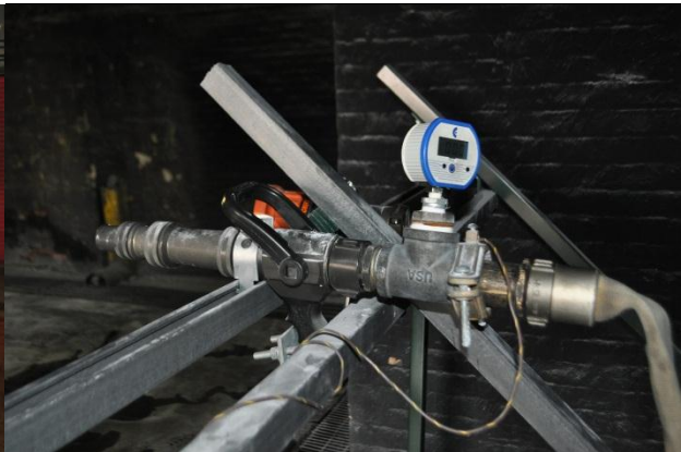
Figure 7 Electrical connection to hose fitting
