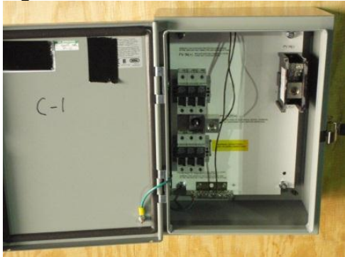
Figure 18 Combiner Box C1 Open
